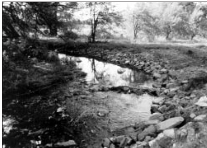
Deflectors in streams concentrate or redirect water flow to restore meandering streams.
